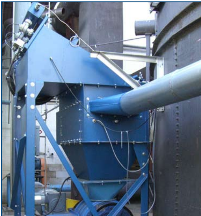
Torit PowerCore at Anderson Corp.
